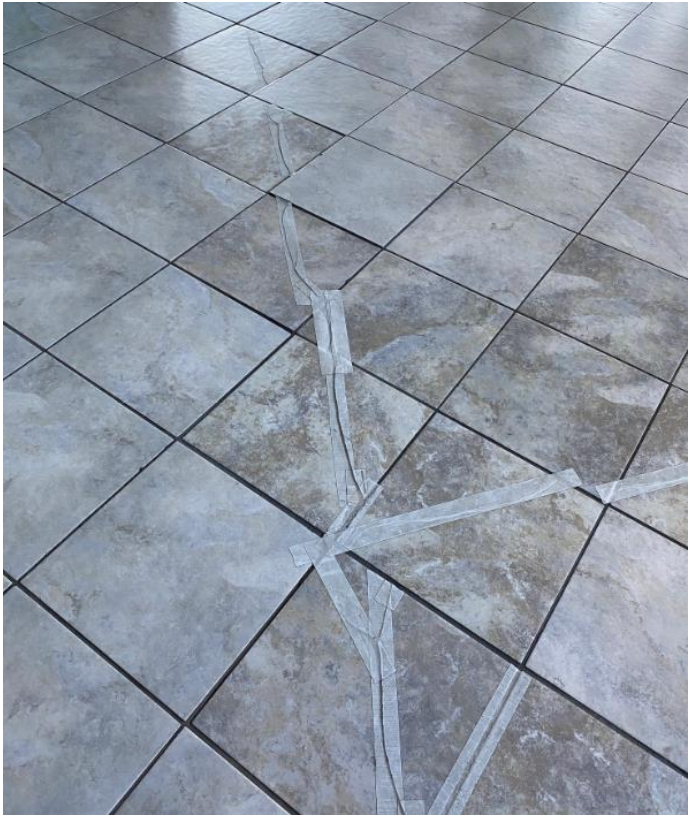
Figure 2: Front Lobby Tile Cracking
