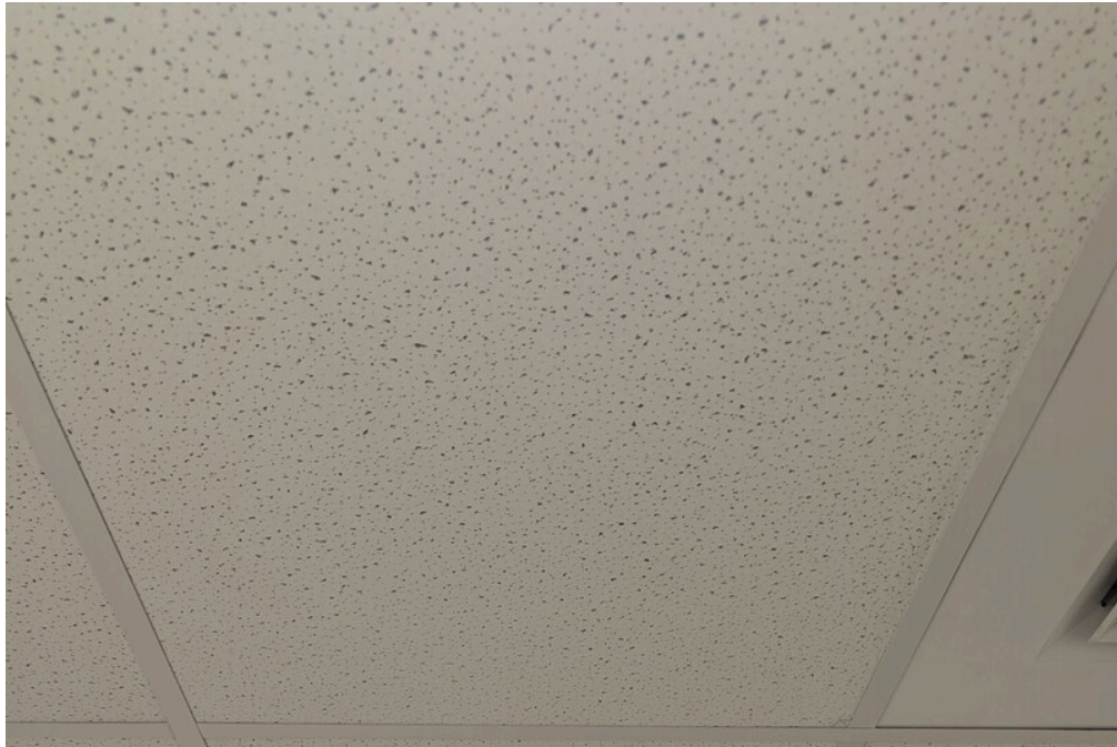
Photo 4: HA03: 2'x2' White Pinhole Ceiling Tile
