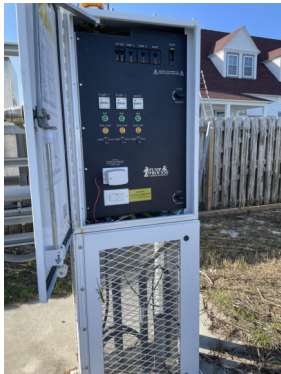
4 PUMP CONTROLLER E301
