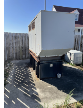
3 EXISTING DIESEL GENERATOR E301
